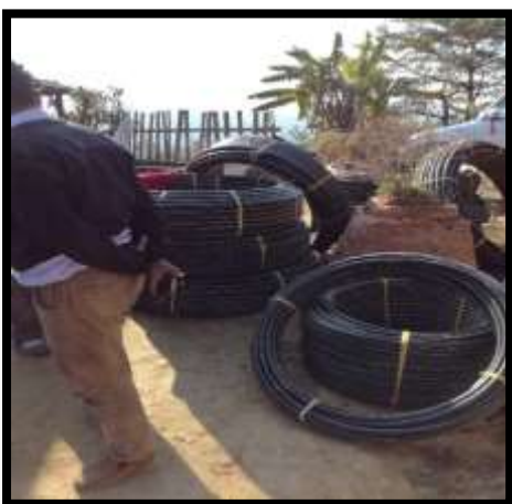
Pipe stored for drinking water supply
